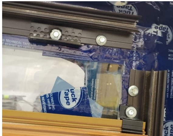
Photo No. 12 Fastener locations at top corner
